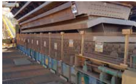
SCREEN FEEDING IRON ORE 4000tph
