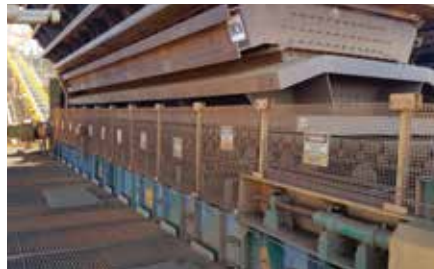
SCREEN FEEDING IRON ORE 4000tph
